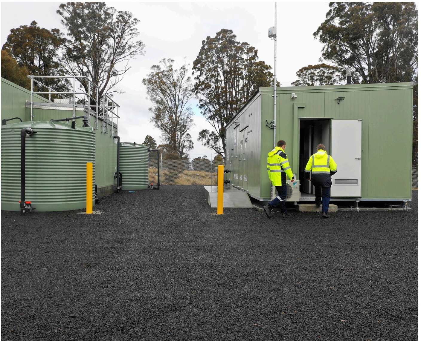
Below: Modular water treatment plant in Tasmania
