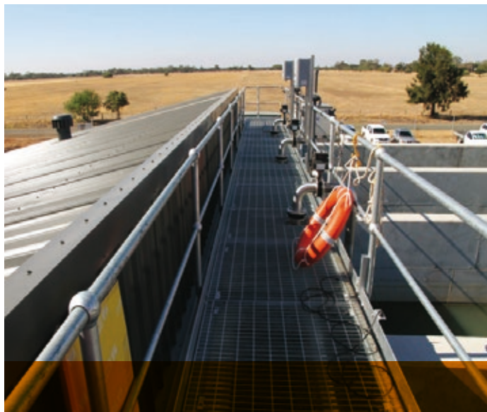
Phase 2 of the BOOT scheme provided effective wastewater treatment, enabling the decommissioning of the original lagoon system. The plant is a modular configuration which is scalable to meet future demands and can be easily configured to produce Class A.
