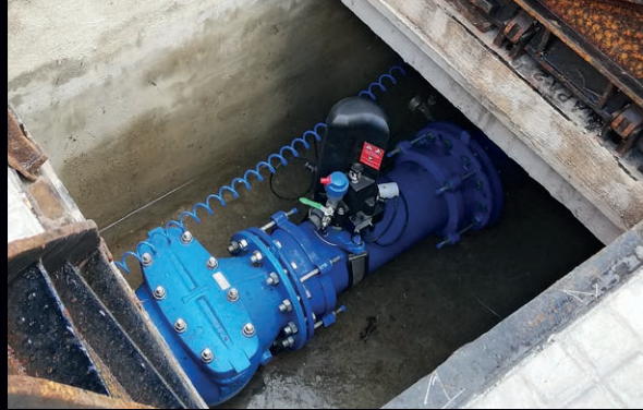
Example of an Installation in a Manhole
