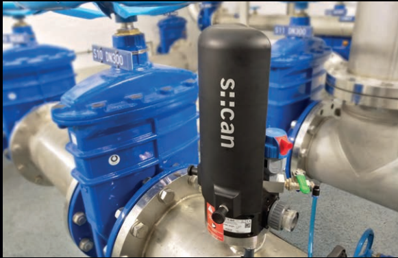
Drinking Water Network Monitoring for Smart Cities
